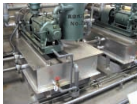
Wastewater recovery facility
